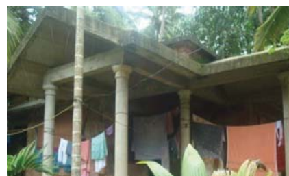
An unfinished house which did not adhere to plinth area limitation
