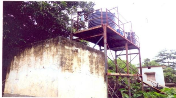
Photograph of non-functional Phoobhanga MRPWSS of Sahibganj
