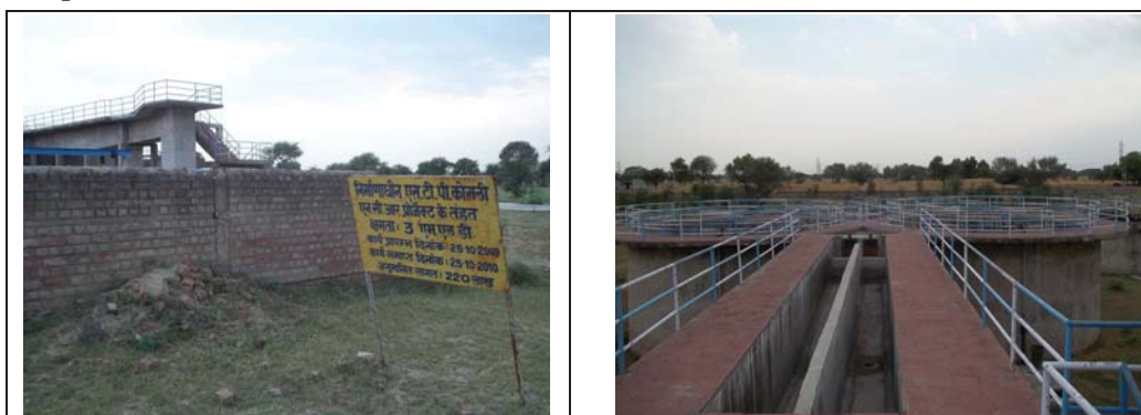
Unutilized three MLD STP at Kosli due to incomplete main sewer line joining STP and non-availability of land for outlet disposal channel carrying treated domestic wastewater (2 April 2013)
