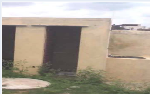
School: Primary school Gram Panchayat: Sirigiripur Thanda Mandal: Maheswaram District: Rangareddy Toilets not in use due to non-availability of water
