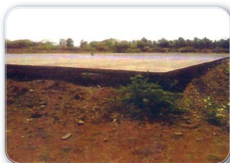
Picture 14 Incomplete VCP at Jafrabad NP, Amreli District (04.06.2013)
