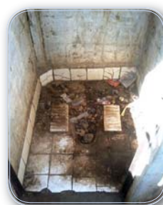
Picture 3 Toilet seat in Kamboi PS, Dahod (02.04.2013)
