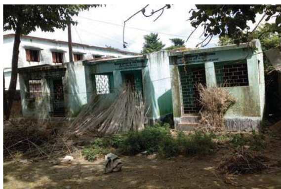
Unused kitchen cum store in Sitalpur Mubarakpur High School, Chanchal-I due to inadequate kitchen space
