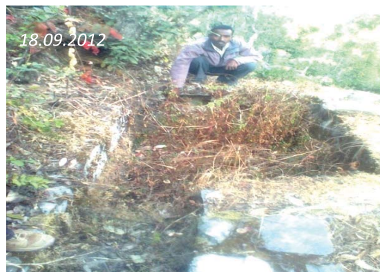
Non-functional Sarna Canal
