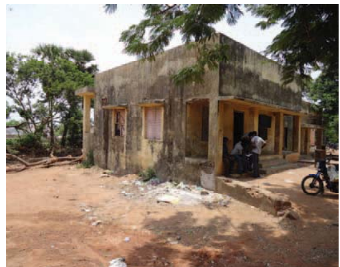
ITI operating in a dilapidated building
