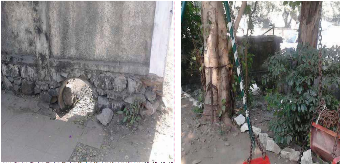
Holes noticed at the base of the compound wall on the front side
