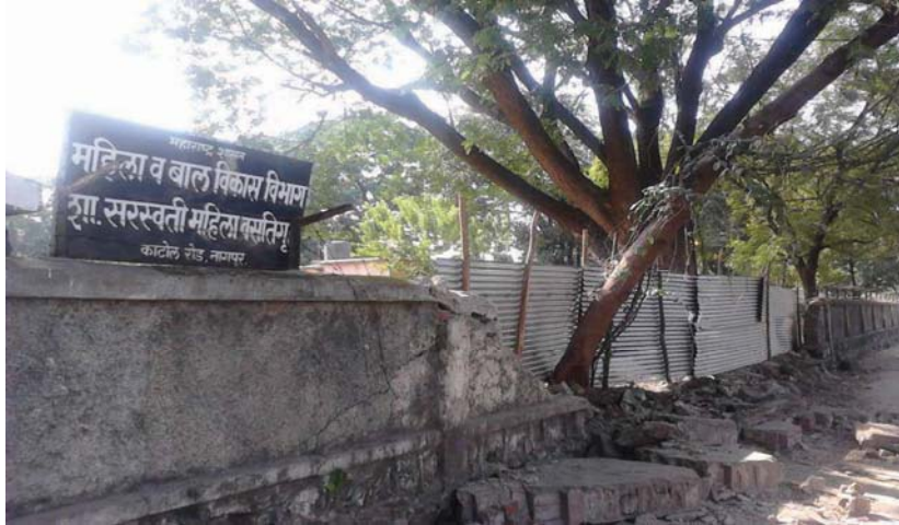
Condition of the compound wall on the front side
