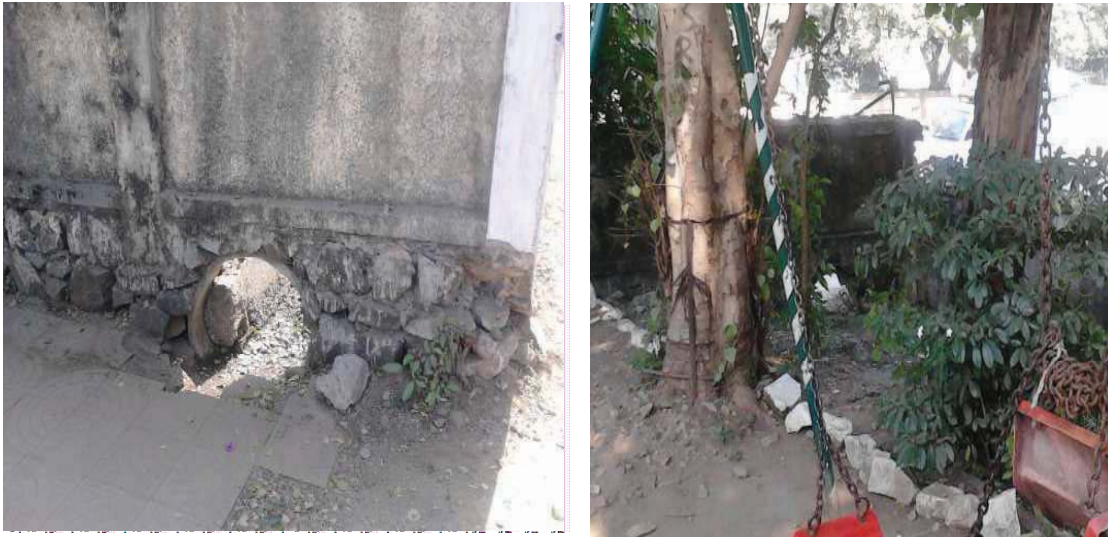
Holes noticed at the base of the compound wall on the front side
