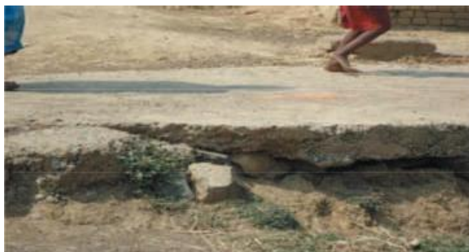
Photograph showing sub standard PCC road at Sitapahari GP in Pakur district
