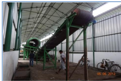
Solid Waste disposal plant not fully in operation (05/06/2012)
