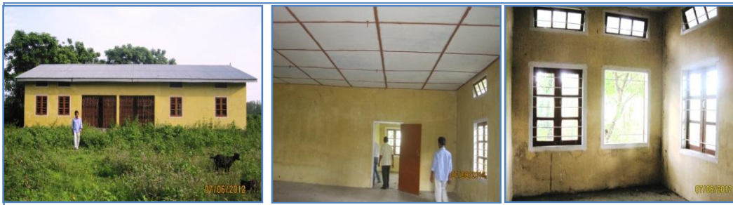
Chicken hatchery without electrification and incubator/machinery was not installed at Biswanath Chariali (07/06/2012)
