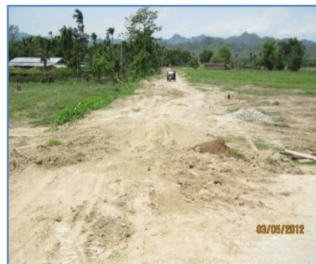
Incomplete road of Solengi to Rajabari via Tinalibari Sonapur to Rajgarh road (03-05-2012)
