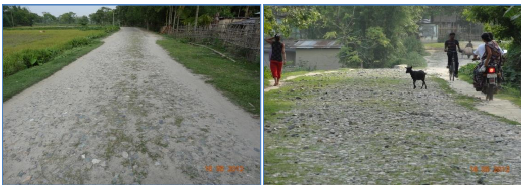
Incomplete PMGSY Road-Tulip Bagan to Rubbar Tola-Package No. AS-22-73 (16/5/2012)
