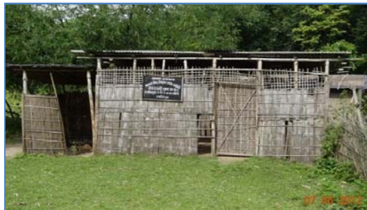
Dilapidated condition of Anganwadi Centre No. 42 at Dhekiajuli (07/06/2012)
