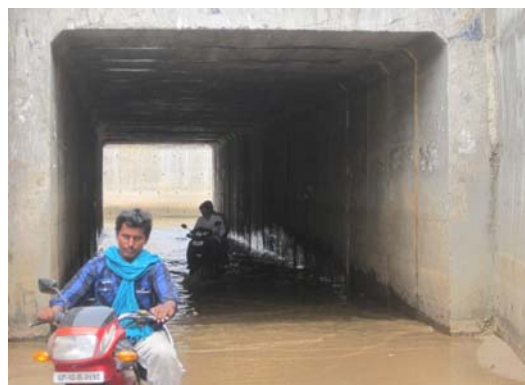
Photograph showing water stagnation resulting in obstruction to traffic at RUB at Puttur Town
