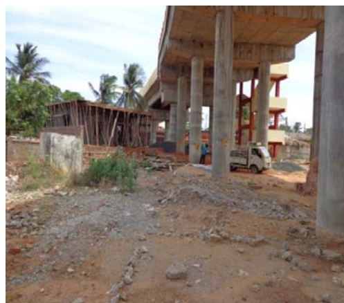
Extra height of bed blocks added by Railways to match height of deck slabs at ROB at Anaparthi
