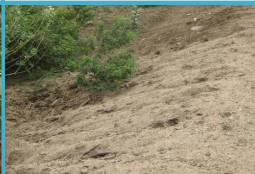
Work ID: 121712613012010417 GP/Mandal/District: KK Agraharam/Bukkarayasamudram/Anantapur Expenditure incurred: ₹44,984 Weakening of bund, due to soil erosion
