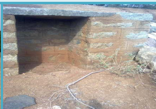
Work ID: 232935613011050110 GP/Mandal/District: Varkala/Chintapalli/Nalgonda Expenditure incurred: ₹16,61,684 No sluice was constructed and the opening was closed by construction of a wall
