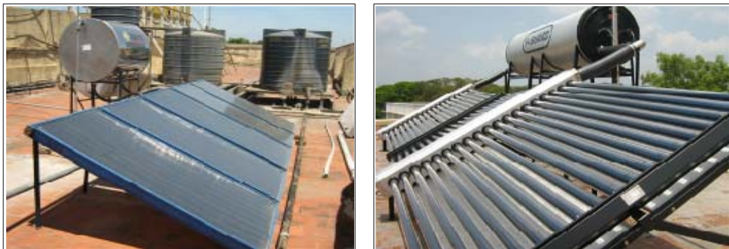
Different types of solar water heaters provided at Tiruchhchirappalli,SR
