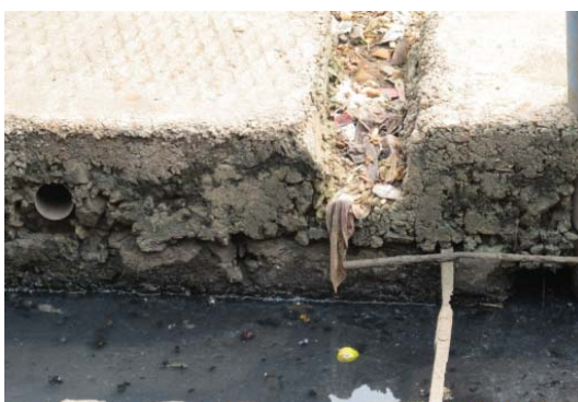
Discharge of waste water from Kharagpur Station (SER)
