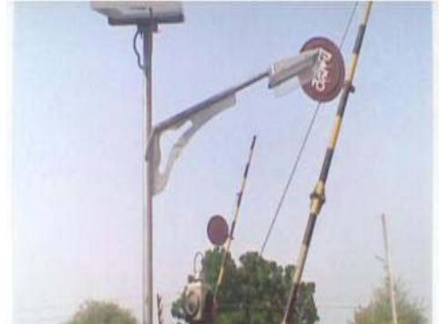
Solar Panel at manned level crossing between Darazpur - Mustafabad section, NR
