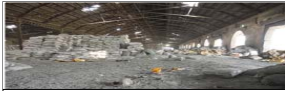
Cement dust at Salt Cotaurs Goods shed, Chennai
