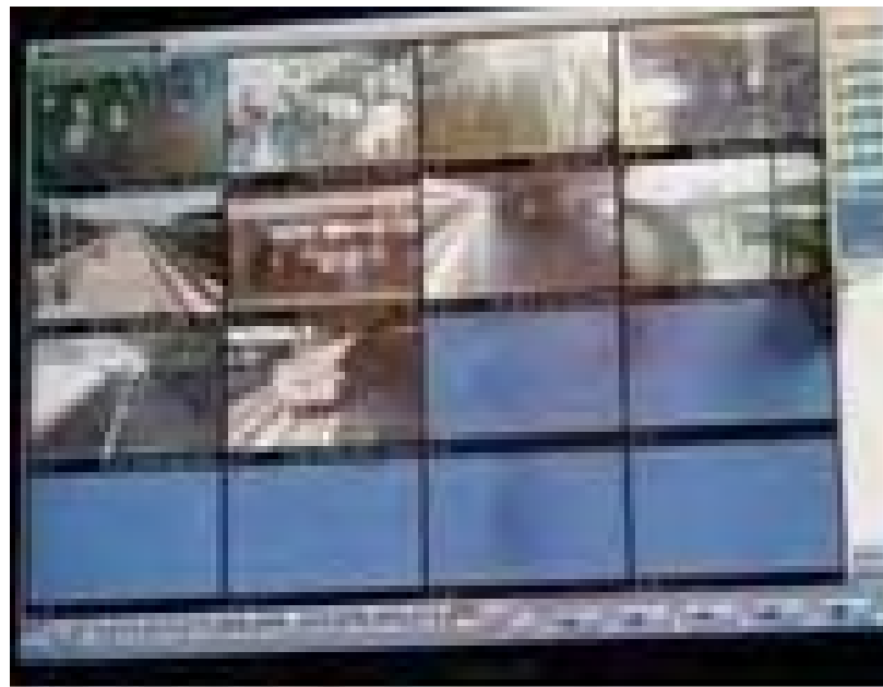
Some of the CCTVs not working at Bangalore in SWR
