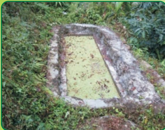
Defunct vermin compost pit under Namphing GPU
