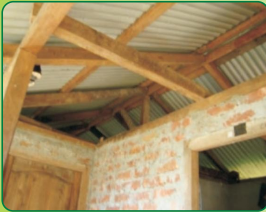
Incomplete RHS at Poklok Denchung GPU
