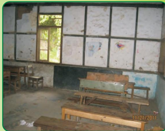
Dilapidated condition of classrooms of Lingmoo SSS under Lingmoo GPU
