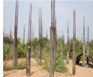
Interrupted construction work of Kalamandal building on a disputed land at Bhubaneswar
