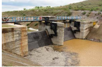
View of additional cross regulator at RD 49.10 km of RBMC obstructing the Water way
