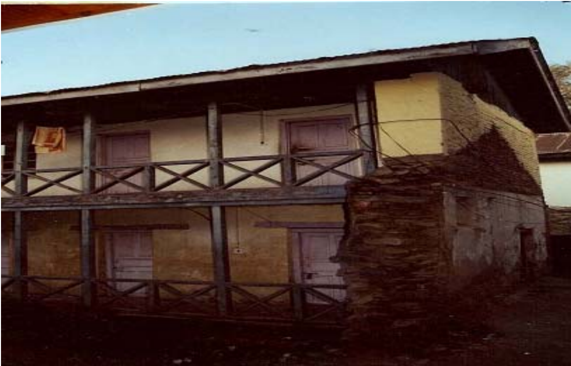
Damaged view of LSQ Baramulla
