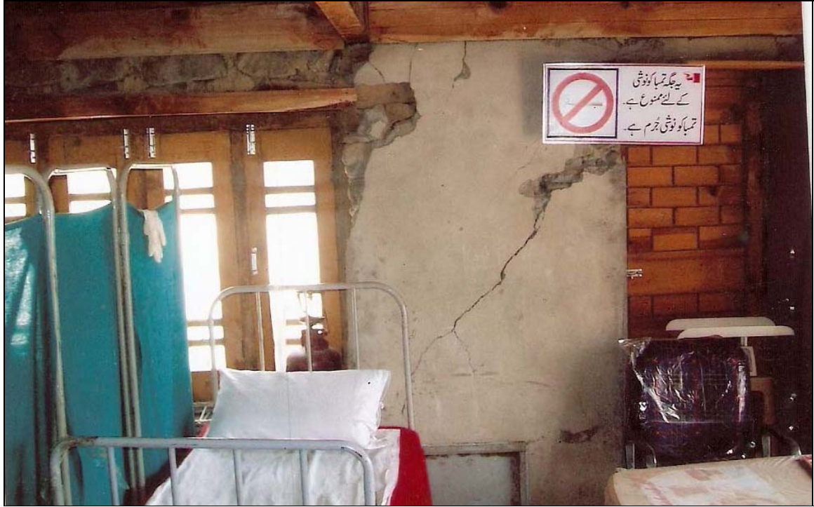
Sub Centre Pheli Pora full of cracks
