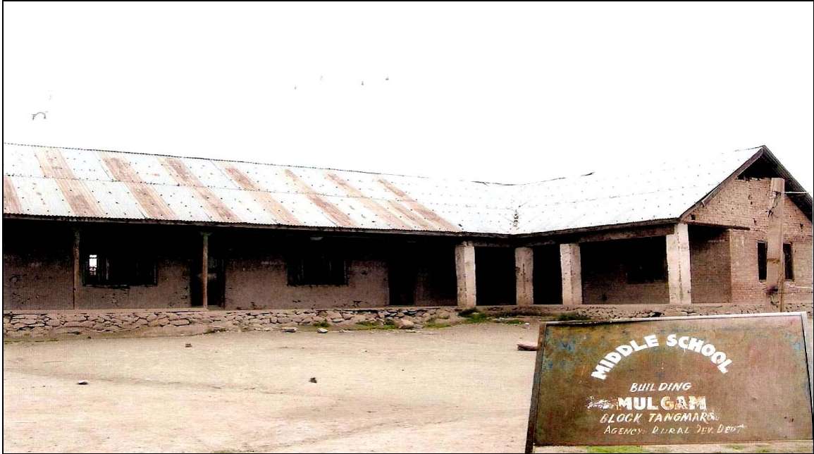
Unsafe building at Mulgam Kunzar
