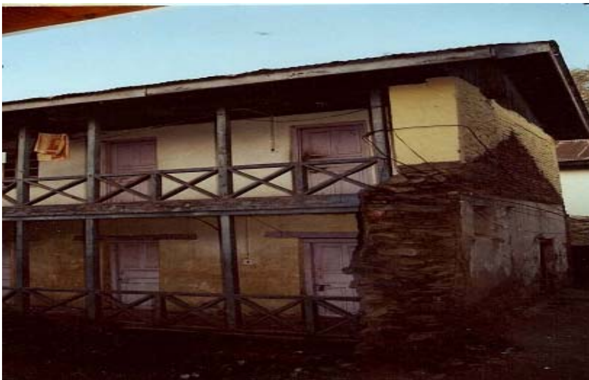
Damaged view of LSQ Baramulla
