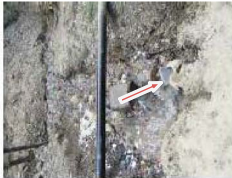
Broken sewer line below IGMC & Hospital (8 February 2011)
