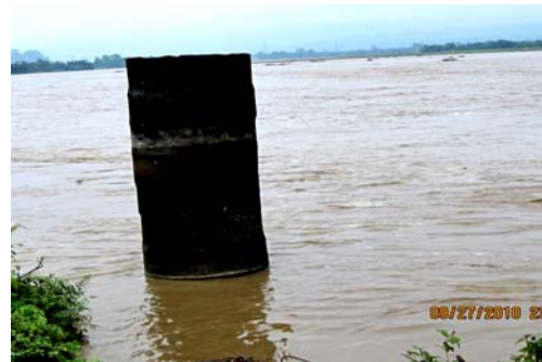
Ring well of a washed away residence
