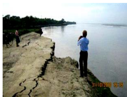
Eroded (breached) newly constructed embankment
