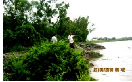
Breached newly constructed embankment
