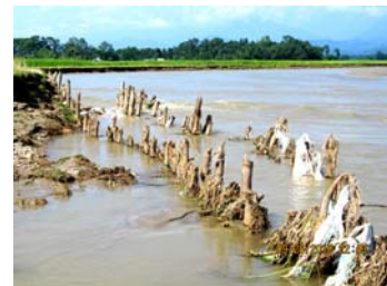
WASHED AWAY COFFER DAM OF KAKOI RIGHT BANK (September 2010)
