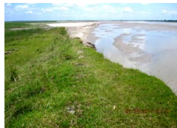
4.2 Km open breach embankment of Jiadhhal river in Dhemaji District
