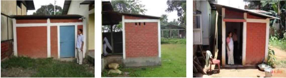
Construction of KSR attached to Main School buildings in violation of norm at (1) Government MV School, Nagaon (01 August 2011) (2) Morigaon Town MES, Morigaon (29 June 2011) (3) Rajdhani LP School, Dispur (16 June 2011)
