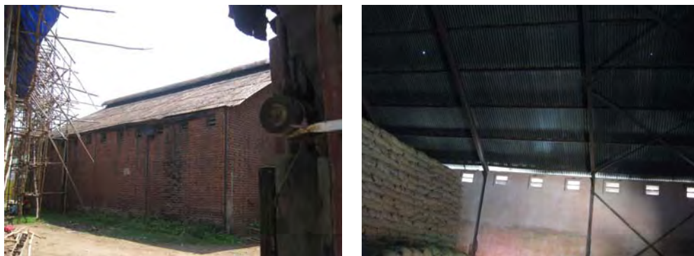
Damaged sheds of Bardhaman-South Food Storage Depot which are yet to be repaired by Zilla Parishad
