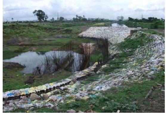
Fig. 2: Incomplete Pumping Station at Chowbhaga
