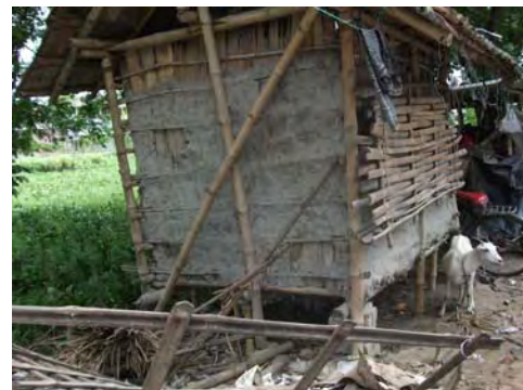
Fig. 1: Encroached Canal Bank
