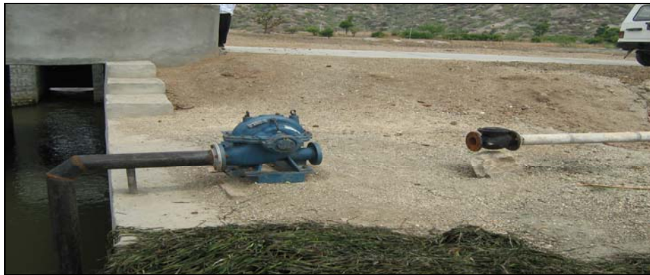
Photograph showing non-connection of rising main of water supply scheme with source (06.07.2010)
