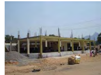
Incomplete bus terminus at Rayagada
