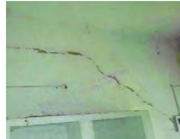
Cracks on the walls of the common room
