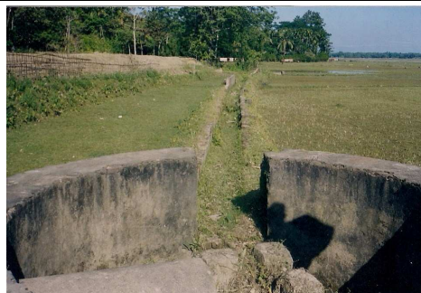
Damaged stilling tank of Gajalghat LIS Phase-I/26 April 2010
