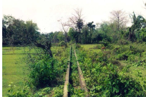
Lined canal of Udharbond ELIS, (Inoperative)/27 April 2010
