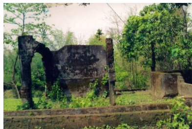
Damaged pump house and stilling tank of Udharbond ELIS, Bagerkona PC (Inoperative)/27 April 2010
