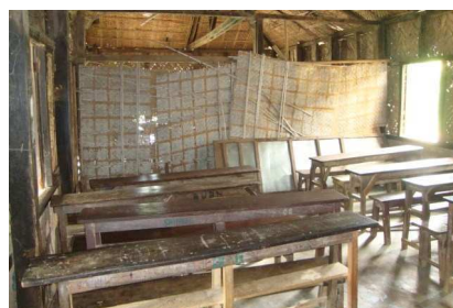
Dilapidated condition of a school/18 May 2010
