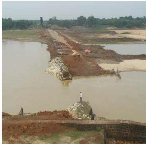
Breached low weir of Anicut after the flood of July 2008
