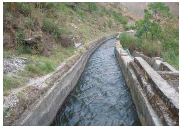
Rajwakti : Uncovered power channel
