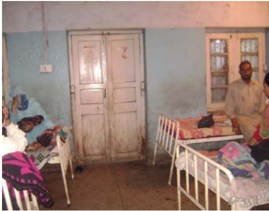
Poor condition of maternity ward at District Hospital, Rajouri, Jammu and Kashmir
