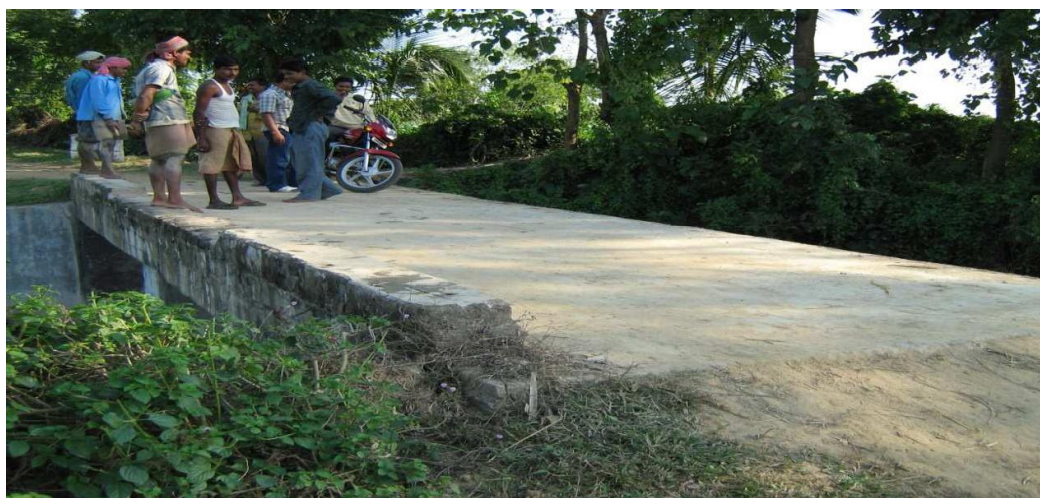
Unguarded Box Culvert at Ishanpur GP causing frequent falling down of cattle.
