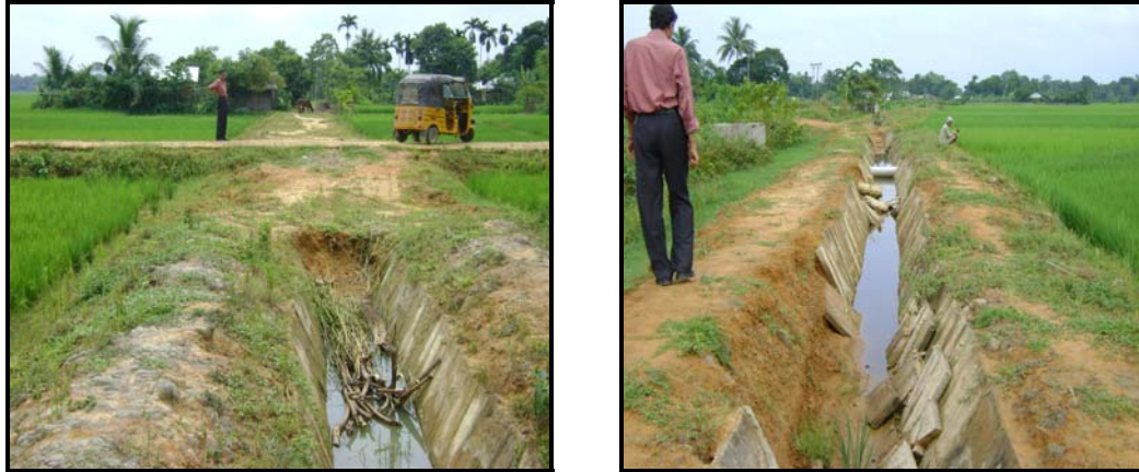
Undeveloped and damaged portions in Khowai Right Bank branch canal breaking the continuity in flow of water
