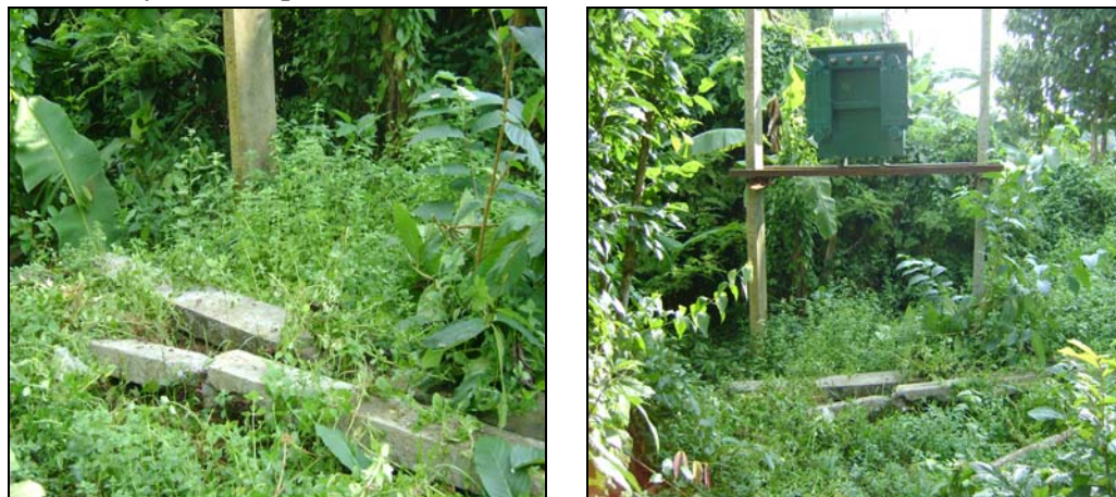
Photograph showing the collapsed pole and reinstalled transformer without energisation
