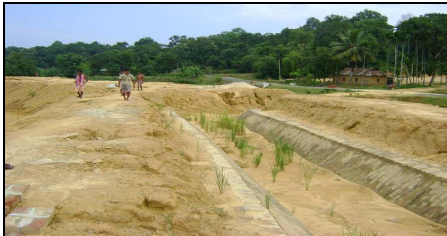
Discontinued Khowai Right Bank main canal due to land dispute and marshy land
