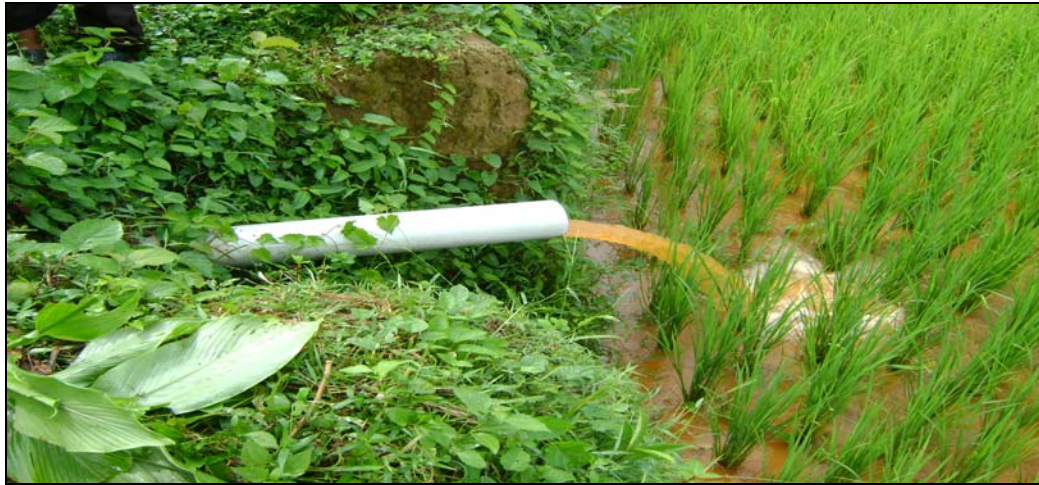
Photograph showing low discharge of water in Nirvoypur DTW scheme
