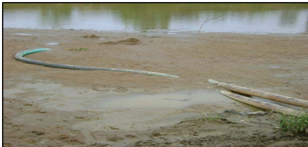
Sand filled foot valve at Bhagyamani Chakmapara LI Scheme
