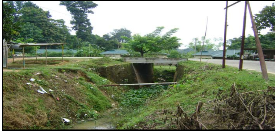
The unexecuted portion of Khowai Left Bank main canal at Reserve Forest Area, Gamaibari
