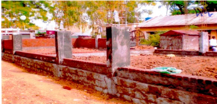
Incomplete work of Government Girl's High School, Molkalmuru
