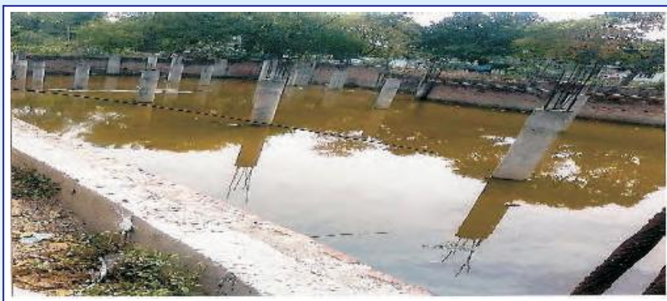
Abandoned work of Parking-cum-Community hall Paonta after incurring expenditure of Rs 39.18 lakh
