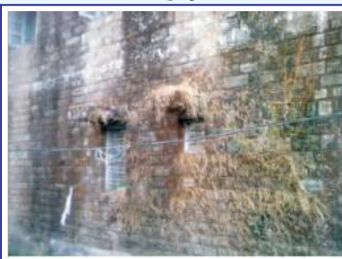
Building of CHC Rajpura covered with wild growth
