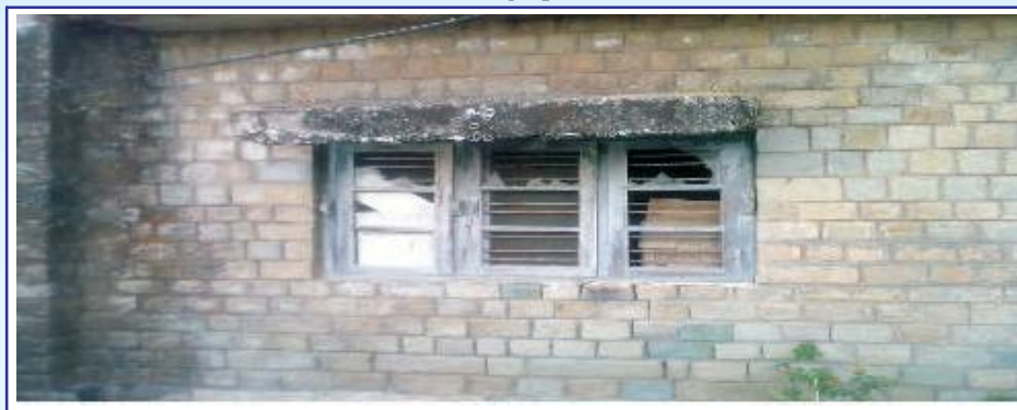
Dilapidated condition of operation theatre at CHC Rajpura
