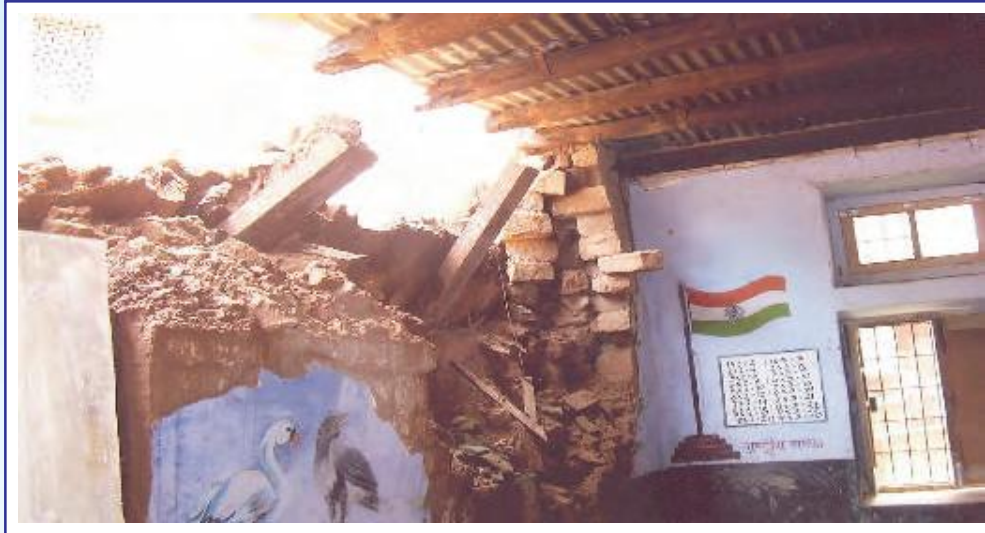
Classroom in GPS Barachowk Nahan in a dilapidated condition
