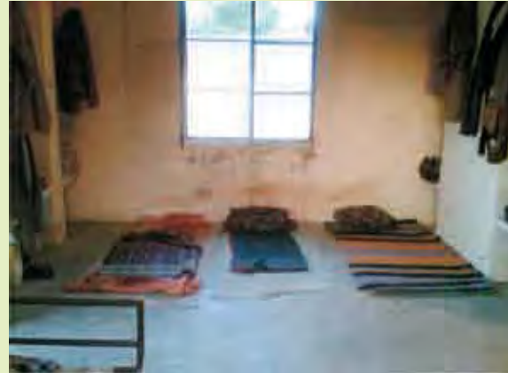
Rest room for males at PS Amb without any basic facilities like attached toilets, baths, cots, bedding, etc.
