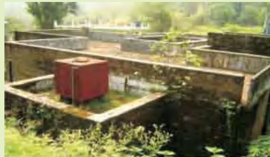
Dilapidated condition of residential facilities for staff CHC Bhota
