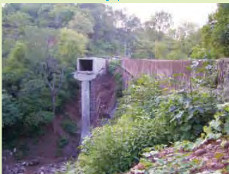
Aquaduct at kms 6.867 to 6.909 kms lying incomplete due to slow pace of work by the contractor
