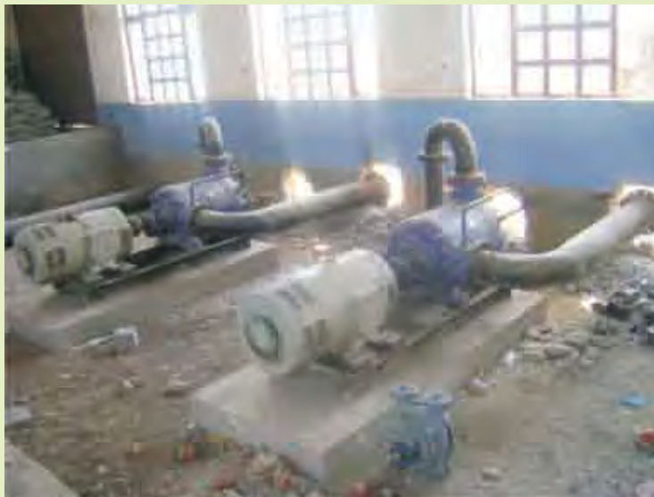
Pumping machinery of zone 1D awaiting supply of power
