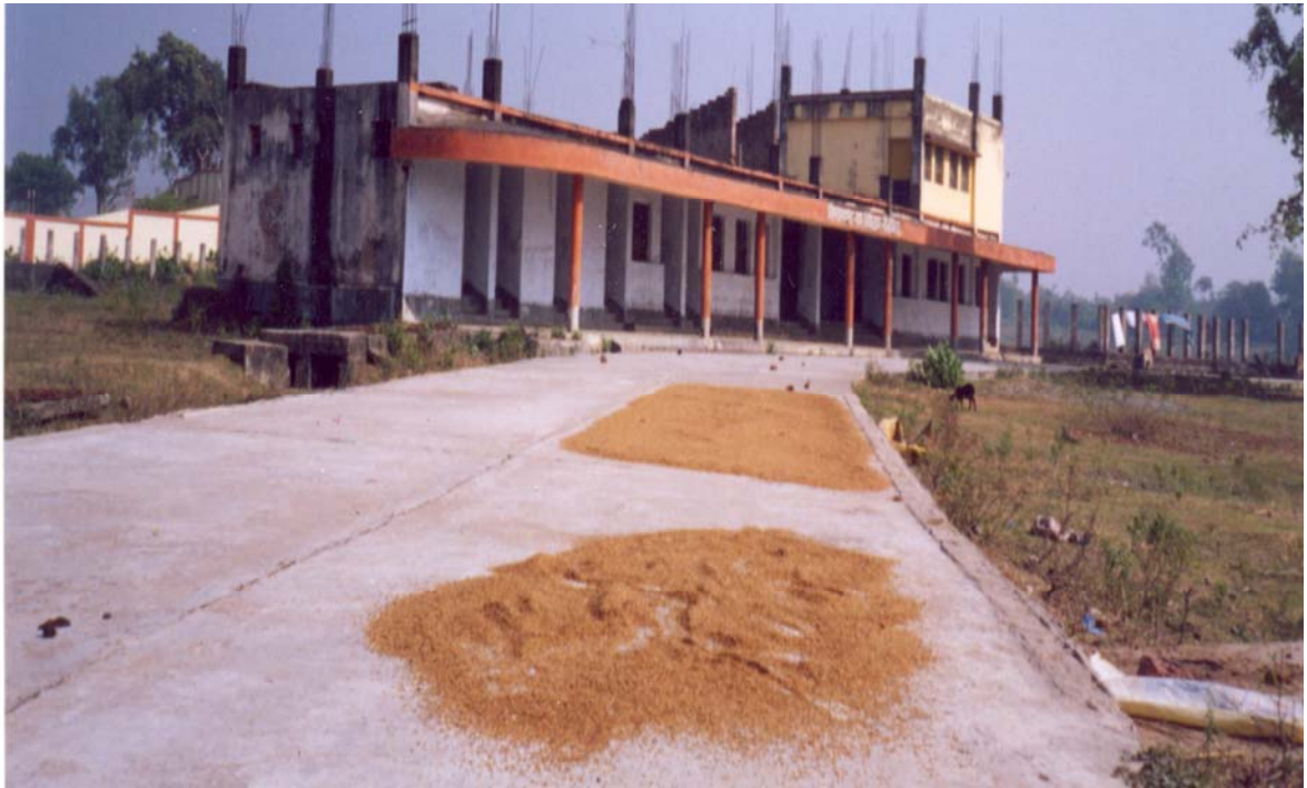
The concrete pavement of the incomplete Vidyasagar Bus Terminus is being used for drying boiled paddy.
