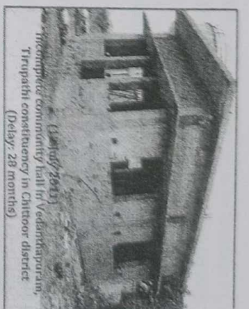
(11 July 2011) Incomplete community hall in Kothamreddy, Pithapuram constituency, East Godavari district (Delay: 25 months)
