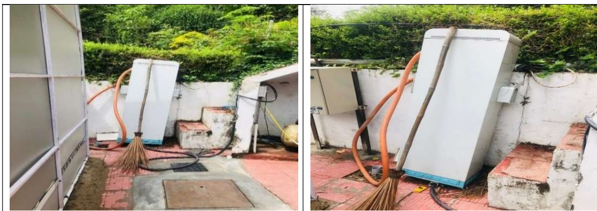
Picture 2: Sawhney Automobiles, Solan, Himachal Pradesh Chargers removed from installation site
