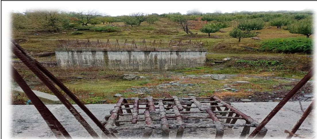
(Bridge at Wahidina Bandi Payeen over Khrus Nallah to which approach roads were yet to be constructed)
