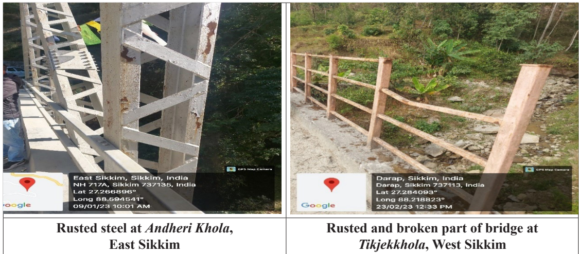
Image 3.20 & 3.21: Rusty and broken bridge parts due to maintenance
