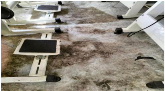
Image 2.6: Discoloured marble flooring
