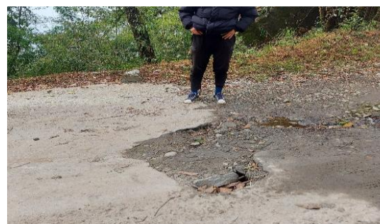
Damaged culvert wall and slab
