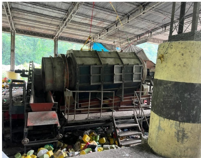
Image 7.21: Non-functional Processing facilities
