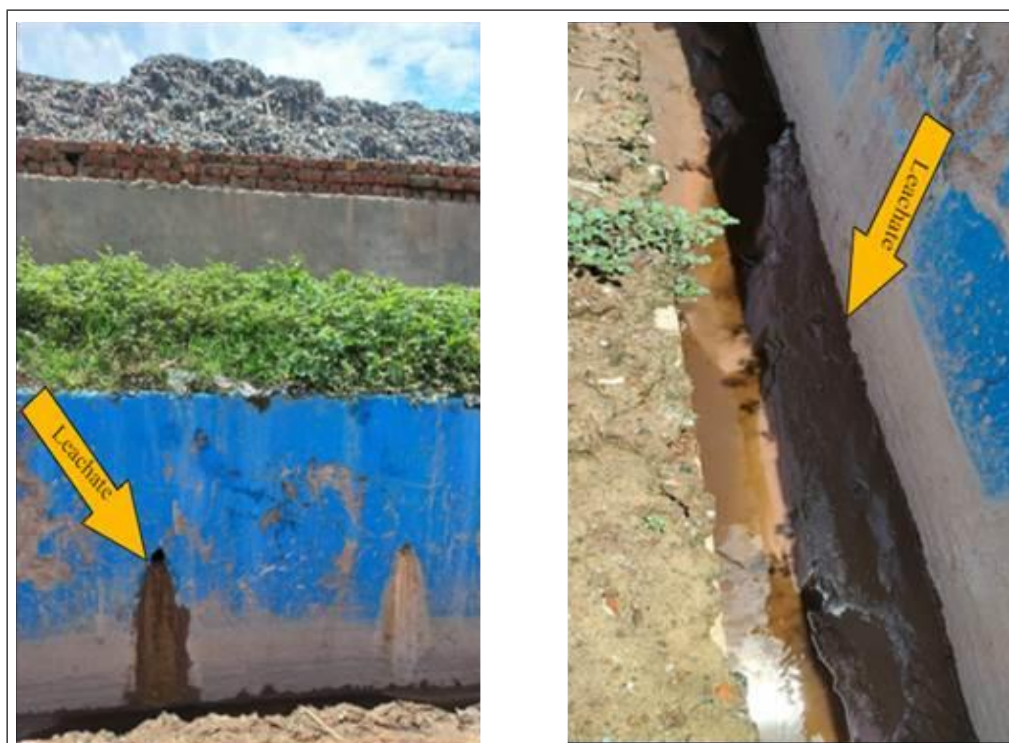
Figure 6.1: Leachate coming out of Dhapa dumping yard of KMC
