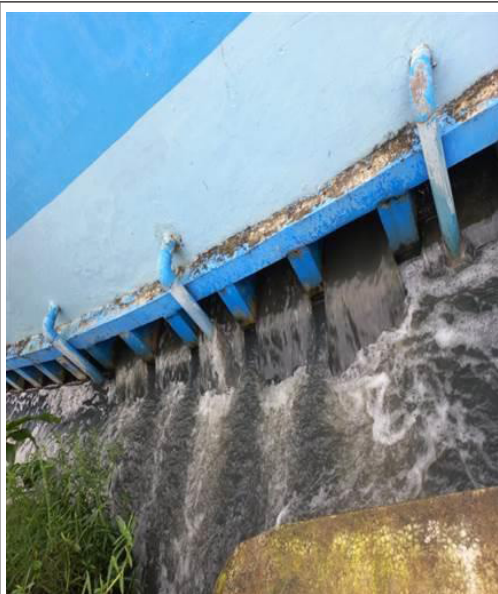
Figure 4.17: Treated water discharging into outlet drain
