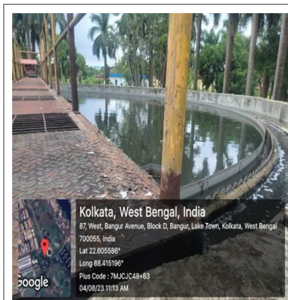
Figure 4.16: Primary Clarifier at the STP
