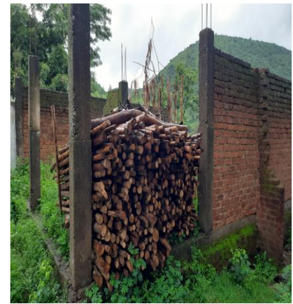
Picture 5.13; dated 10.07.2023 Incomplete Classroom inside the premises of Renu Project Upper Primary School
