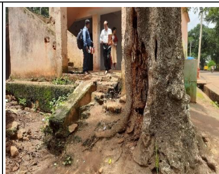
Picture 5.10; dated: 13.07.2023 Unsafe ramp/ entrance to Classes VI and VIII at Hataguda Upgraded High school
