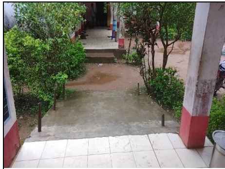
Picture 5.9; dated: 12.08.2023 Ramp with broken angle in Pendapada Primary and Upper Primary School
